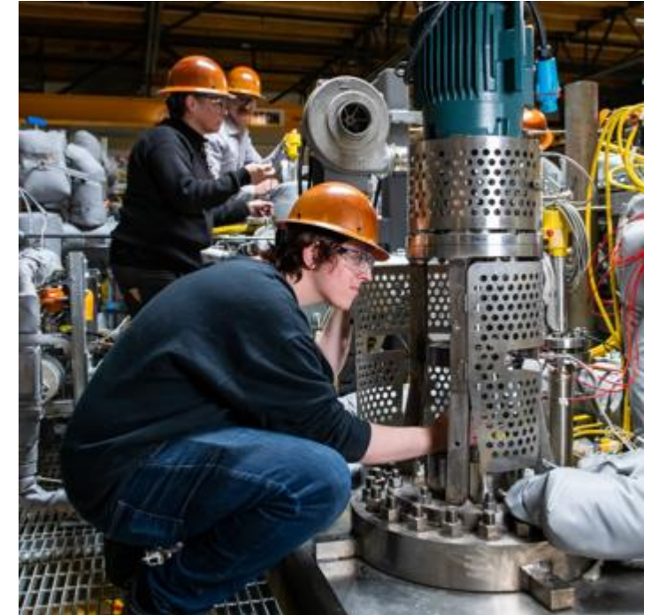
TerraPower technician with HT molten salt pump
